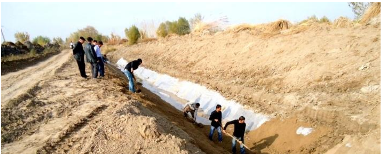
After draining and levelling the channel, community members lined the channel with a PE film to avoid leakage
