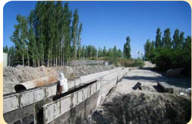
The construction of the canal for the micro hydropower station led by Rahmatullo Shodiev in the Ok Machit village.
