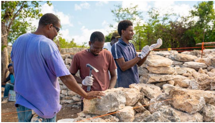
Team restoring the dry stone wall at Owny Well (Photo courtesy Chaso Media)
