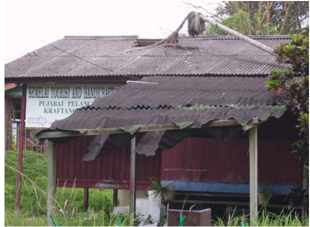
SABOT office in need of repair after tree fell on rooftop
