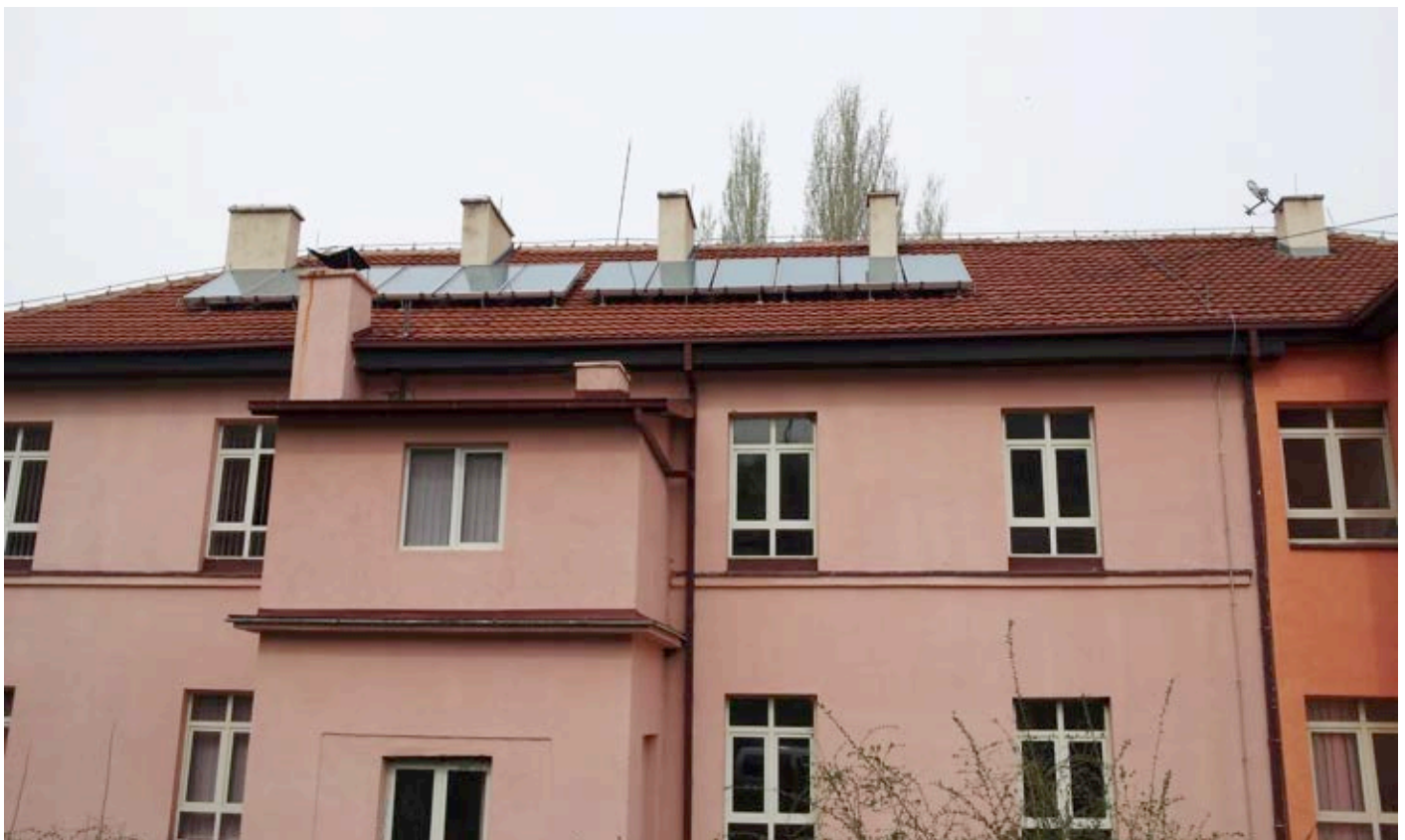
Solar collector in the school Sinisa Stoilov, Zrnovci, photo Zaklina Golceva
