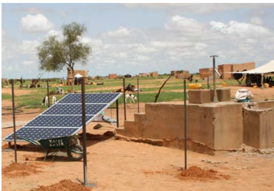
Seenou Kuna Solar Pump, Mauritania
