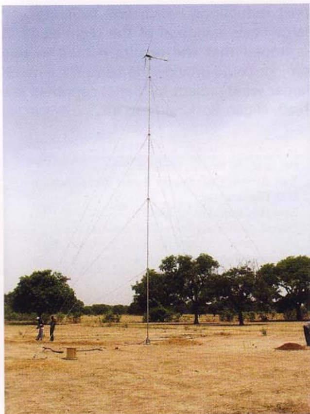
A 1kW wind turbine was installed on a tower of 20m height to avoid wind obstruction by trees in the area.
